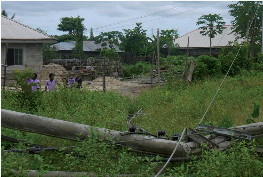
Damaged Transformer Oduoha
